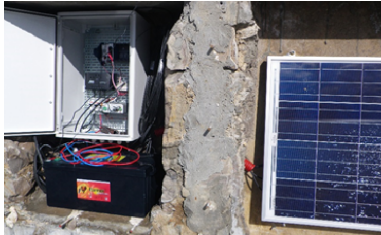
Figure 6: Station de mesure et installation photovoltaïque
