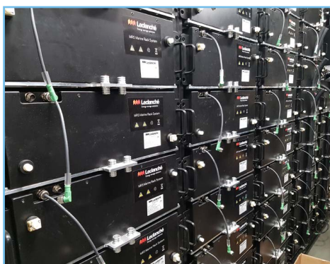
Fig. 12 Battery storage of Li-Ion batteries.
