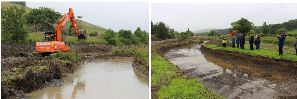
Figure 2.4.2: Remeandering the river channel at Milkiston, in 2016. Left: Gravel extraction, Right: Excavating the new channel, witnessed by some of the team-members from Work Package 4.
