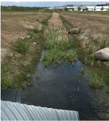
Figure 2.3.2. The two-stage channels design was constructed in 2015. The lack of shading has led to a dense in-channel vegetation.
