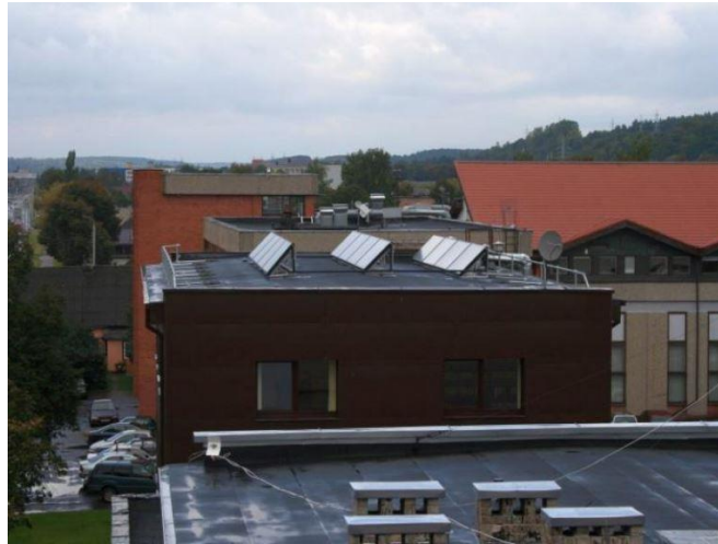
Figure 12. Solar collectors on the roof of the Kaunas DH company building (20.4 kW)
