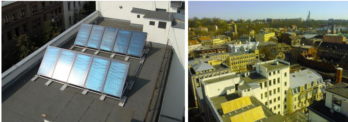
Figure 13. Solar collectors on the roof of the Kaunas City Municipality building
