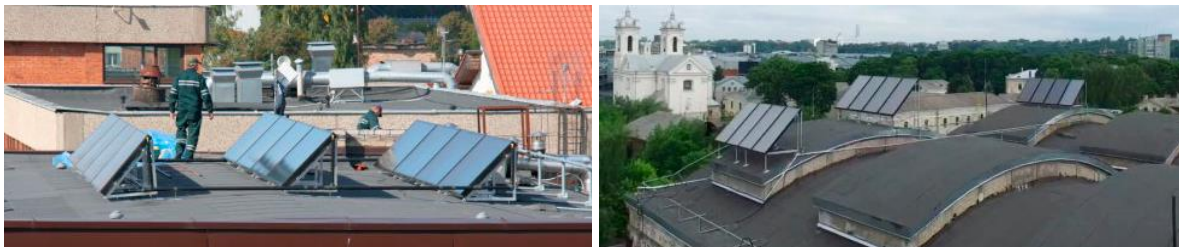
Figure 5. Solar collectors on the building of AB Kauno energija and Pergalė boiler-house.
