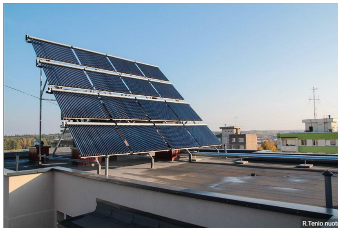
Figure 15. Solar collectors, installed on the roof of residential building Škirpos 15, Kaunas. © R.Tenys photo
