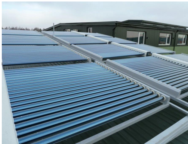
Figure 14. Solar collectors, installed by pharmacy company „Acconitum“ © Company photo
