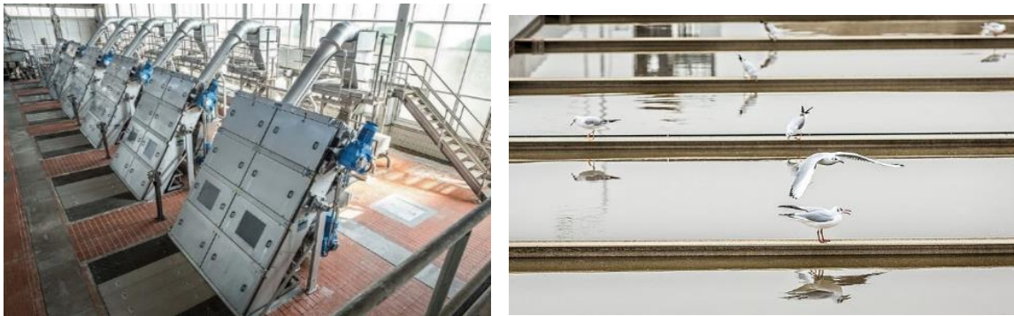
Figure 38: Screening system and primary sedimentation (right) of wastewater treatment plant Vienna (left) (EBS, 2019)
