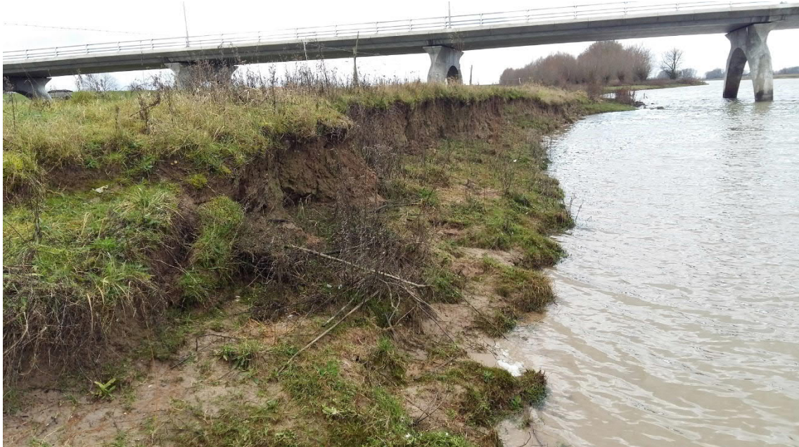
Figure 3.53 Lexkesveer: erosion on the south bank.
