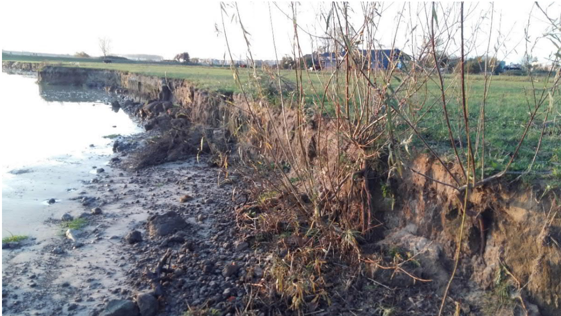
Figure 3.61 Bank erosion in the Pontwaard
