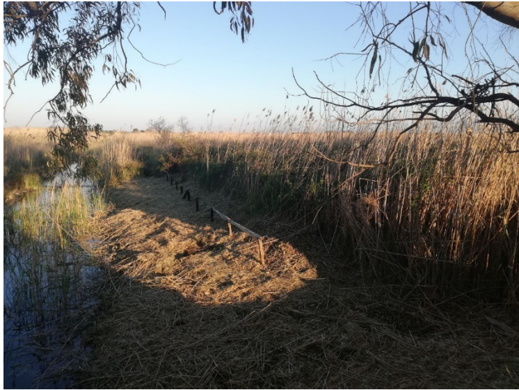
Figure 7: Reed vegetation maintenance works along the channels of the Arneo Consortium that fall within the perimeter of the Reserves
