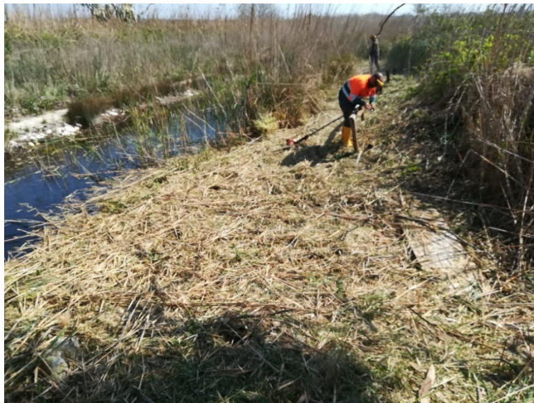
Figure 8: Reed vegetation maintenance works along the channels of the Arneo Consortium that fall within the perimeter of the Reserves
