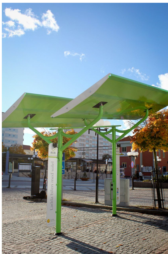
charging station powered by photovoltaic panels installed in the Eskilstuna center in Sweden
