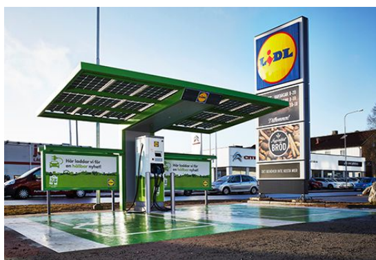
charging station built inside a parking lot of a supermarket in Sweden.
