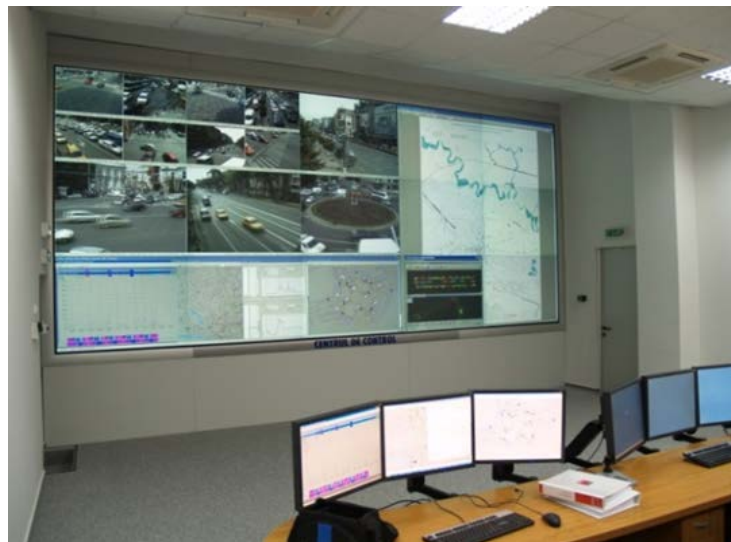
Figure 3-7 Videowall in Bucharest Traffic Management Centre (SWARCO Romania, 2017)
