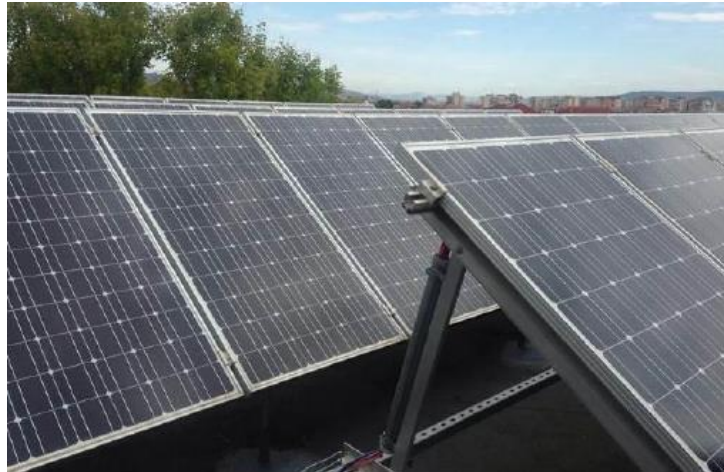
Figure 6 - Solar PV Panels installed on an elderly home at Alba Iulia municipality.
