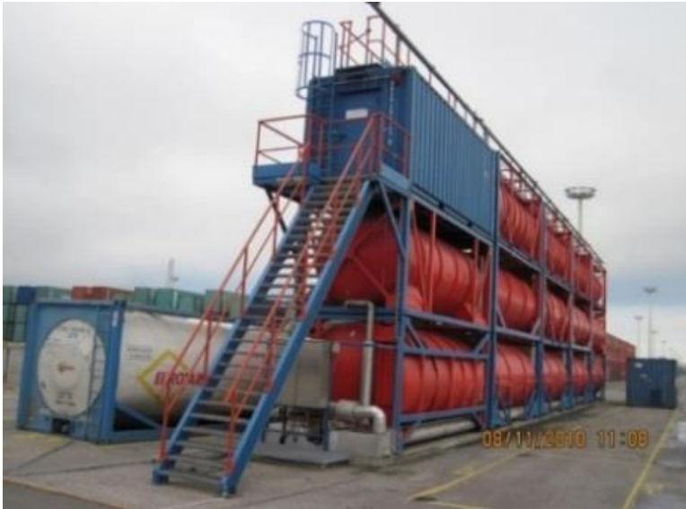
Figure 15: Semi-stationary foam fire extinguishing system at tank container facilities
