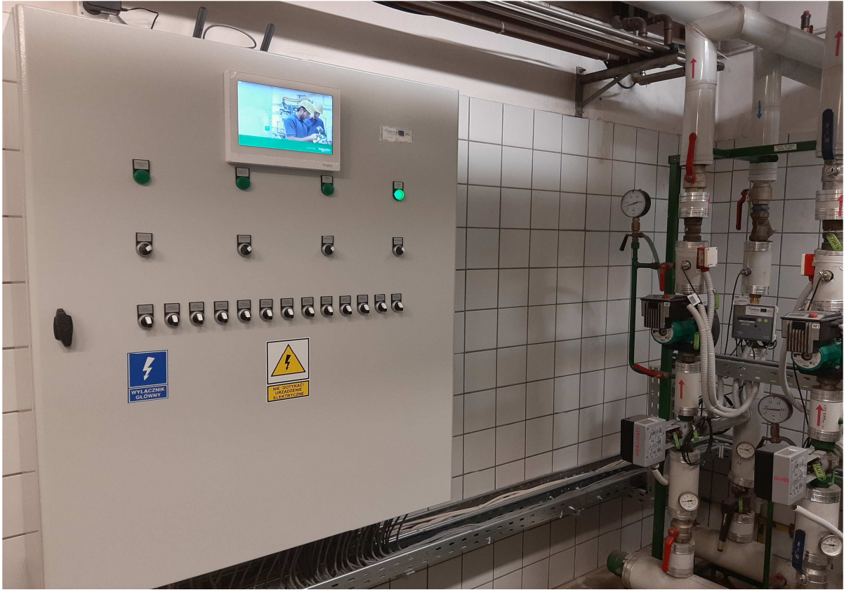
Figure 33. Main panel of the EnMS system installed in the heat node.
