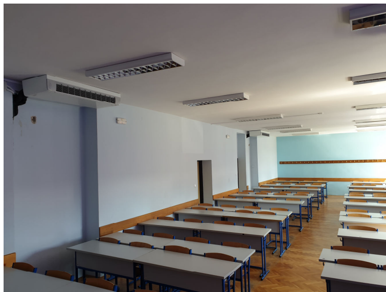
Figure 6.57 Fan converters of thermo-technical system in the UNISB building, G111
