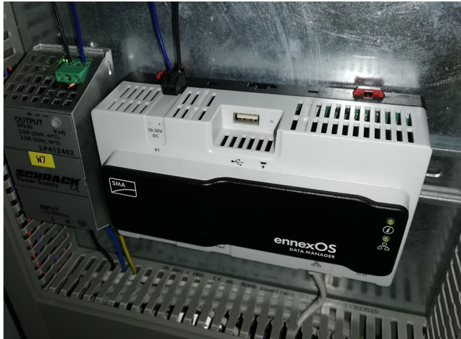
Figure 7.14 KBCO data logger SMA Data Manager M
