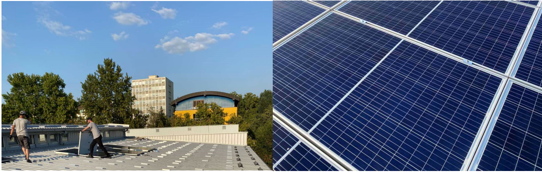
Figure 6.17 PV system on the Emergency center roof
