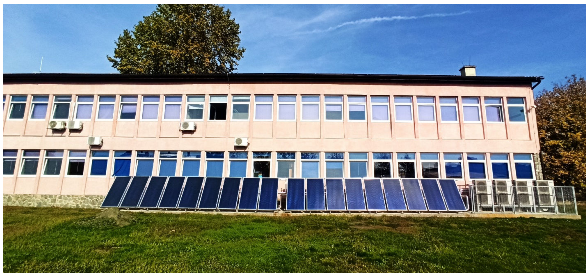
Figure 6.59 Outdoor thermo-technical system of the UNISB building
