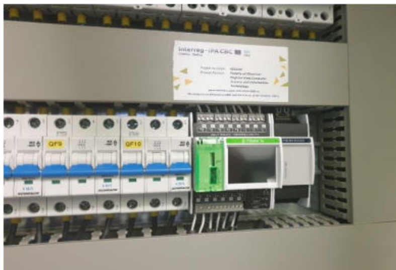
Figure 7.12 PQ3 in electrical switchboard RO-SE2
