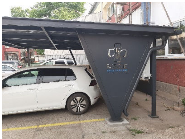
Figure 6.5 Solar powered EV charging station
