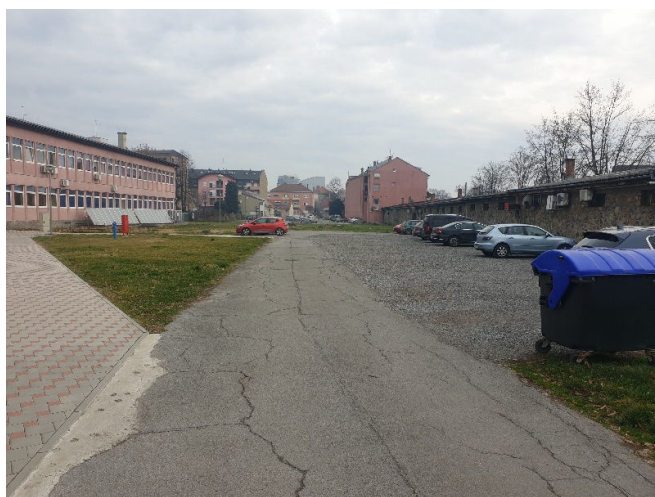
Figure 2.19 Part of Mechanical Engineering Faculty with parking area and installed solar thermal and heat pump's systems
