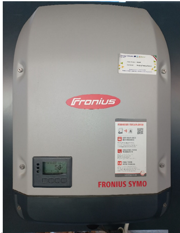
Figure 6.8 The inverter unit that connects PV system for EV charging station to the grid
