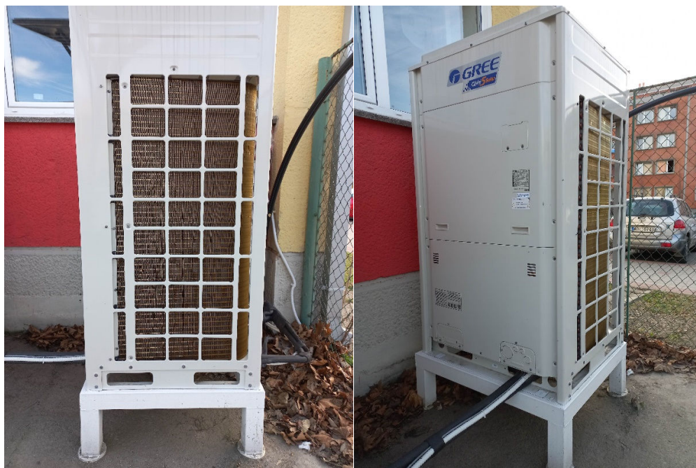
Figure 6.12 Installed HVAC unit
