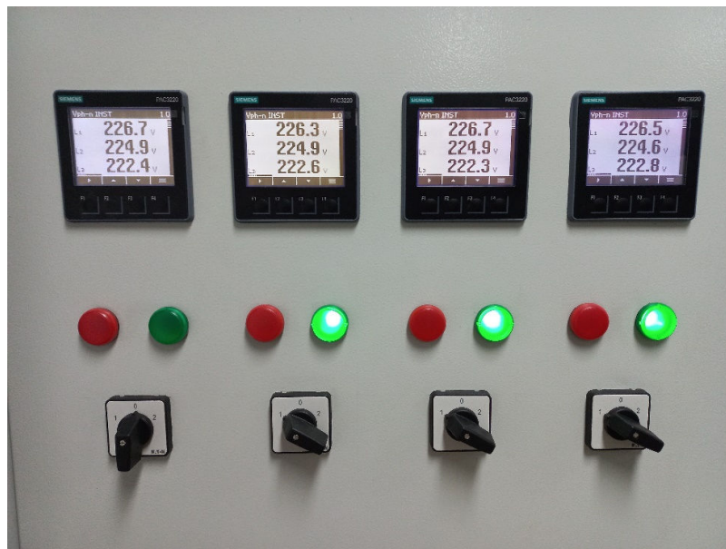
Figure 7.1 Installed Siemens Sentron smart power metres.
