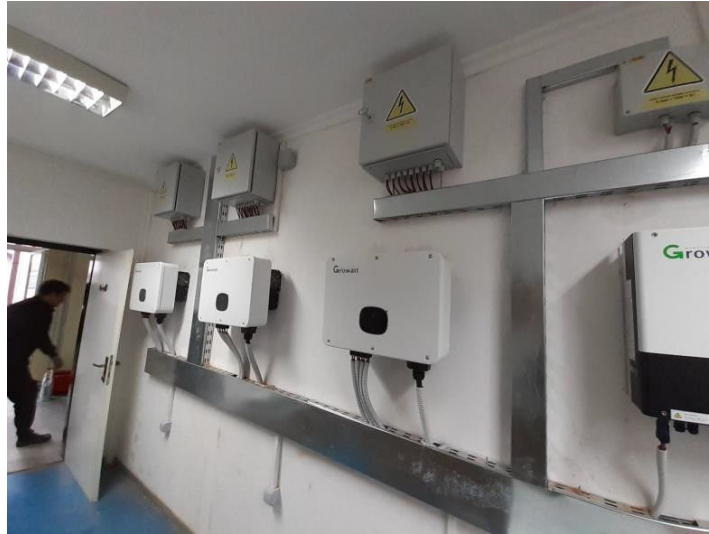
Figure 6.42 Inverters of Photovoltaic power plant on UNISB building in Laboratory for renewable energy sources
