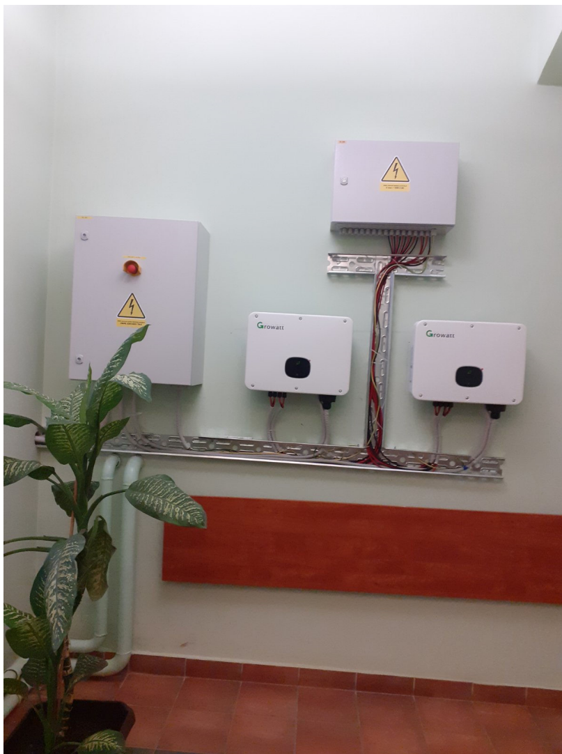
Figure 6.31 Wall-mounted inverters at the 1 st floor of FERIT building in Cara Hadrijana street
