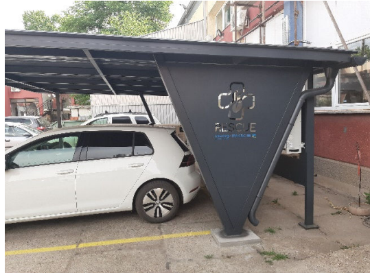
Figure 6.18 PV plant on the KCV parking
