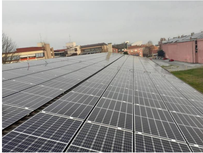
Figure 6.41 Photovoltaic power plant on UNISB building in I. Gundulić Street
