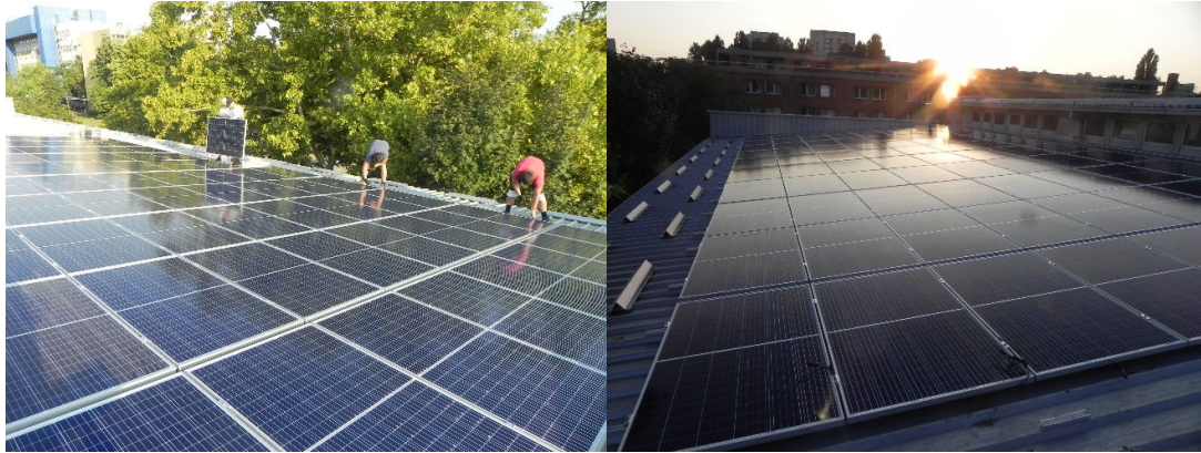
Figure 6.13 PV system on the Radiology clinic roof
