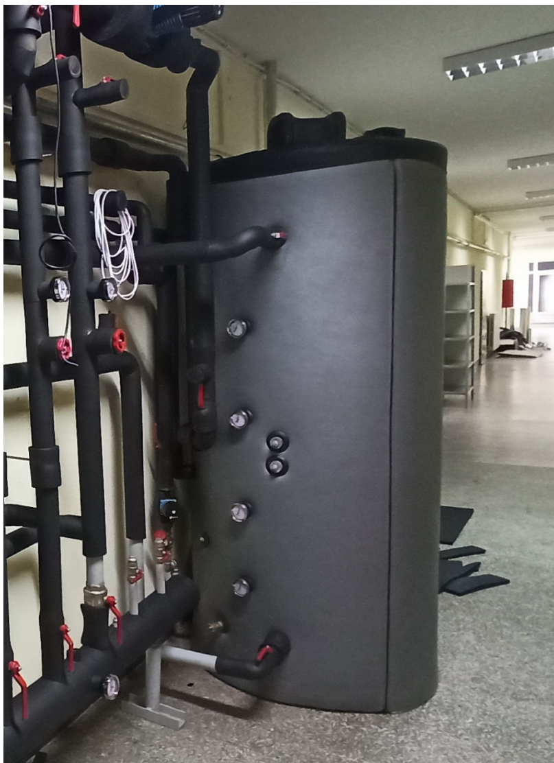
Figure 6.55 Vertical insulated storage tank in the UNISB building
