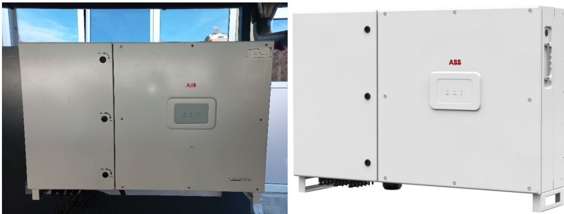
Figure 6.2 ABB solar inverter
