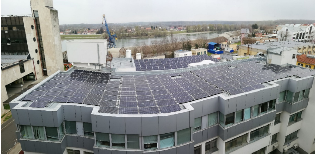
Figure 6.38 KBCO photovoltaic system on Department of Oncology and Department of Diagnostical and Interventional Radiology building roof
