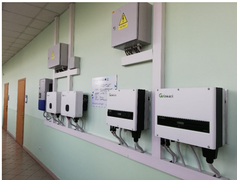
Figure 6.28 Wall-mounted inverters at the 3 rd floor of FERIT building in Trpimirova street
