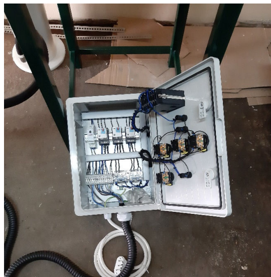
Figure 6.24 Electric cabinet for supplying the bio-diesel production system
