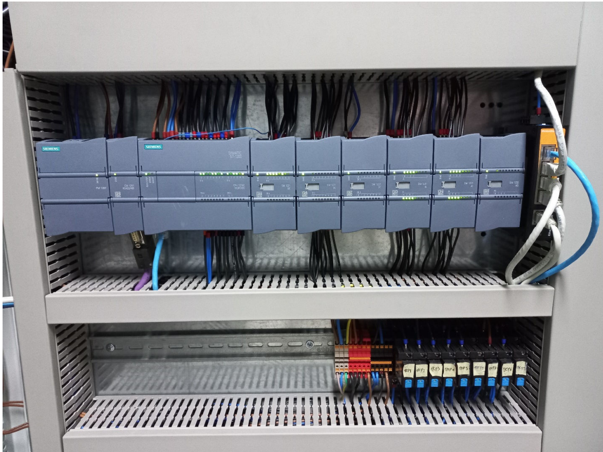
Figure 7.2 Installed PLC unit with additional signal boards.
