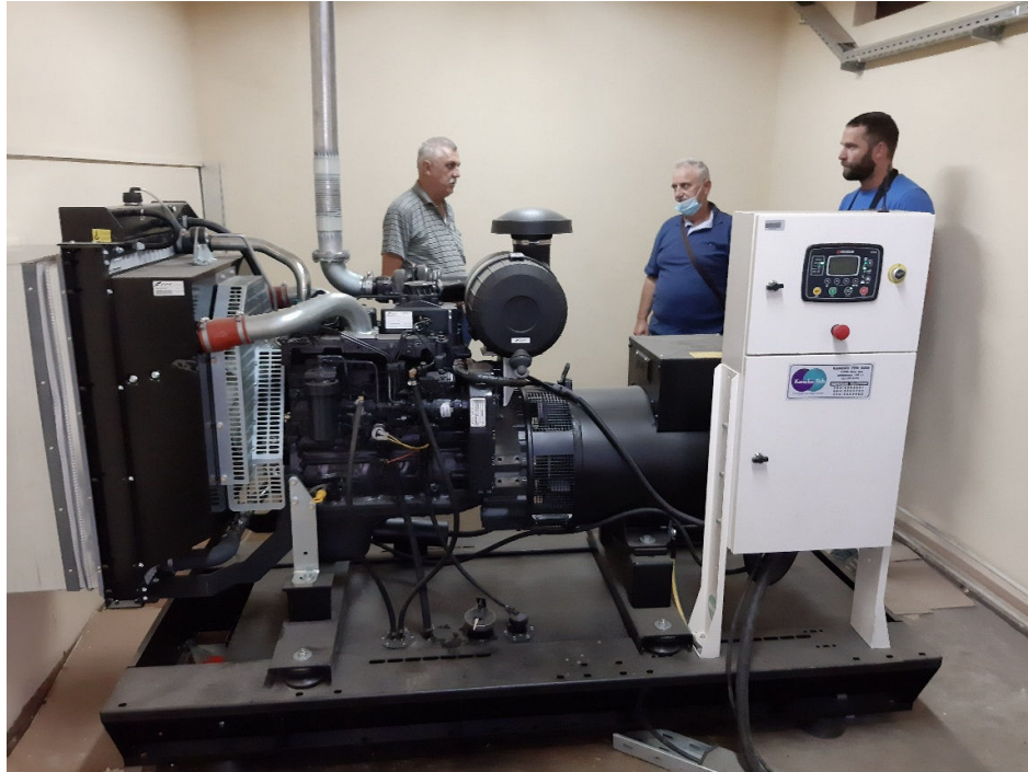
Figure 6.23 Diesel generator system in KCV complex
