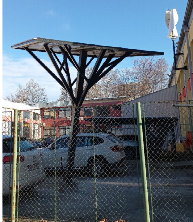
Figure 6.3 Installed solar tree
