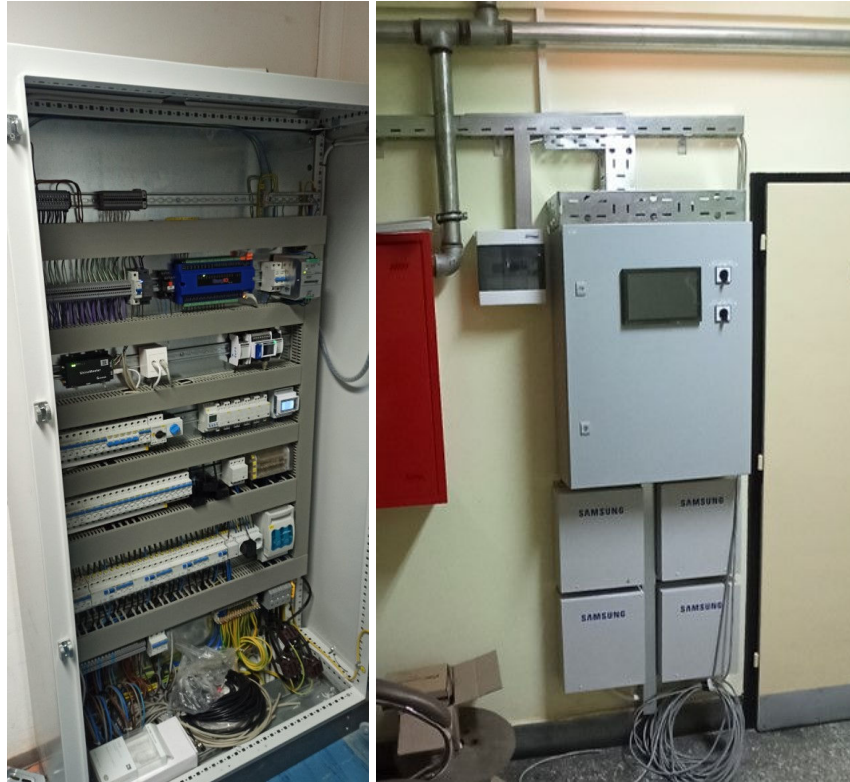
Figure 7.15 Electric cabinets: PV system (left) and Thermo-technical system (right)
