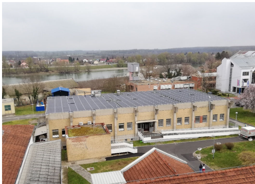
Figure 6.37 KBCO photovoltaic system on central kitchen building roof
