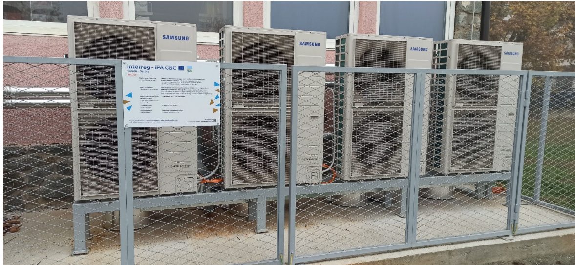
Figure 6.54 Heat pumps installed in front of the UNISB building
