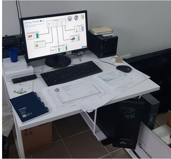
Figure 7.8 SCADA system working station
