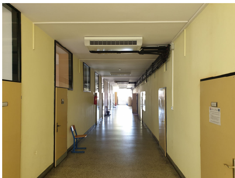
Figure 6.58 Fan converters of thermo-technical system in the UNISB building, corridor
