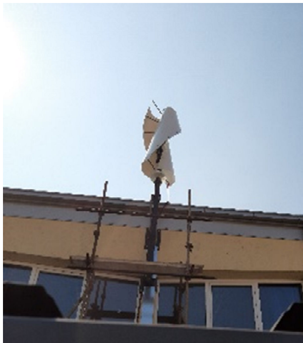
Figure 6.11 Installed wind system at the rooftop of the building
