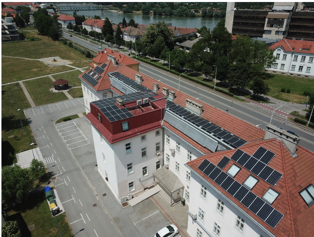
Figure 6.30 FERIT photovoltaic system modules on building roof in Cara Hadrijana street
