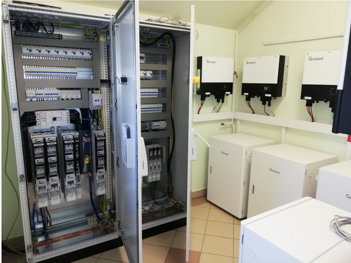
Figure 6.26 Room 3-40 along with RO-SE1, RO-SE2 cabinets and hybrid inverters with lithium battery packs
