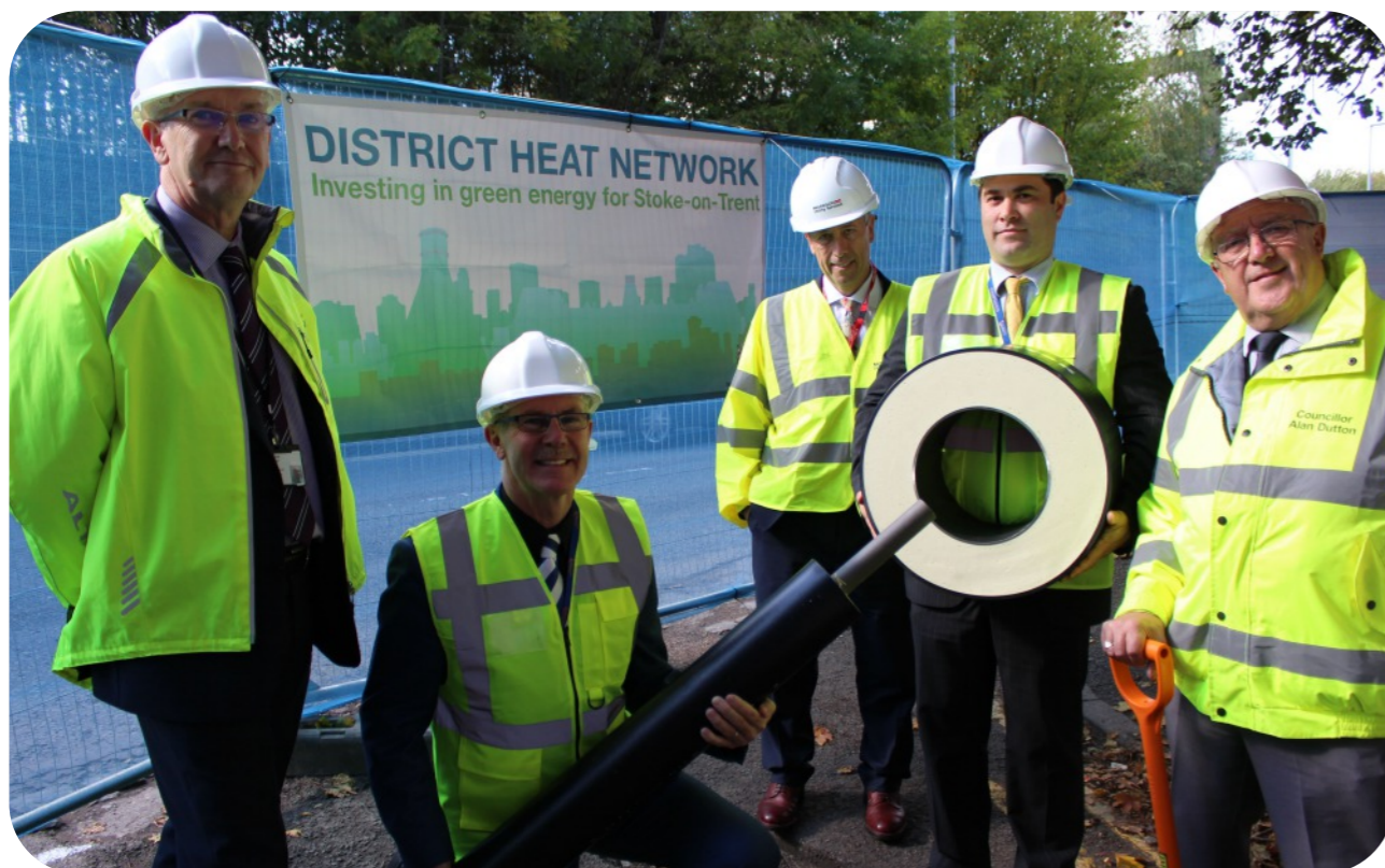
Stoke-on-Trent's district heat network is launched - Pictured (left to right) are: Andrew Briggs, City Council Client Manager - Energy Councillor Anthony Munday, Cabinet Member for Greener City, Development and Leisure Professor David Hawkins, Staffordshire University Dean of Creative Arts and Engineering Sebastien Danneels, City Council DHN Technical Lead Manager and Councillor Alan Dutton, Cabinet Support and Lead Member for the DHN
