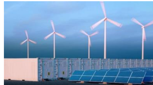
STATIONARY ENERGY STORAGE
