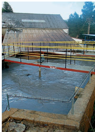
Lime conditioner of the mine drainage
