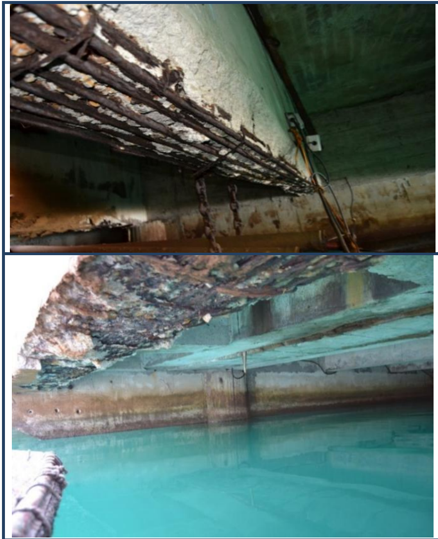
Figure 13: Quay Volujica damages
