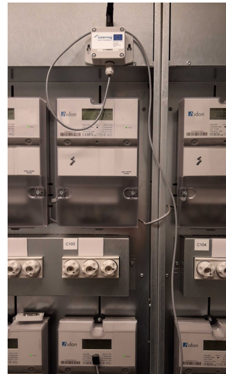
B) LoRa electricity meters
