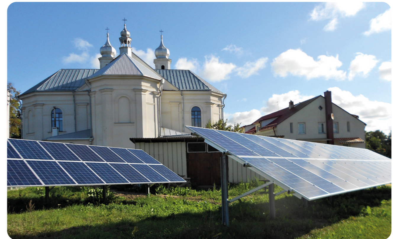
Miroslavas parish 15 kW solar PV supplying the needs of church and community house. Photo by KREA.
