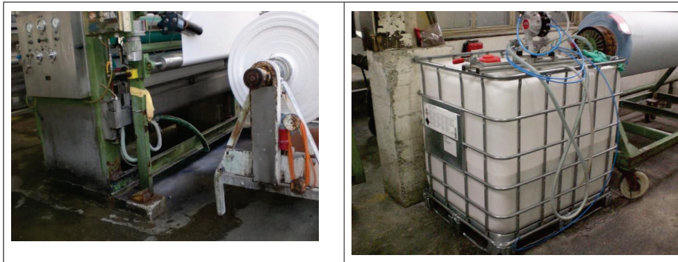
Figure 7: On the left, the photo shows the padder of a stenter and on the right an IBC equipped with a pump and pipes to manually empty the padder (Photos: Dr. Harald Schönberger)
