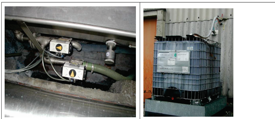
Figure 9: On the left, there is an automated system to segregate the residual dyeing padding liquor and on the right the IBC to collect it (Photos: Dr. Harald Schönberger)
