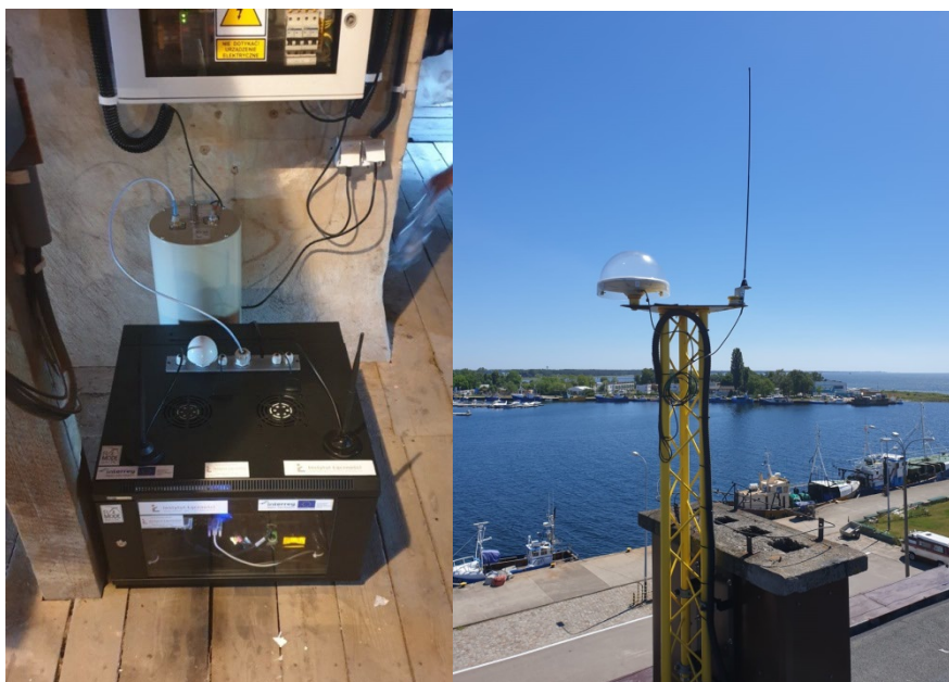
Fig. 6.5 Installation of R-Mode VDES receiver hardware in the port of Jastarnia
