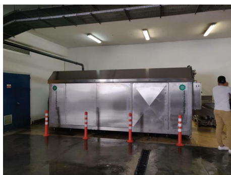
Figure 3: Installation of ACU in the pilot area 1
