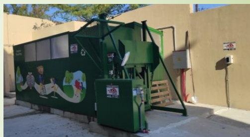
Installed Autonomous Composting Unit (ACU)
