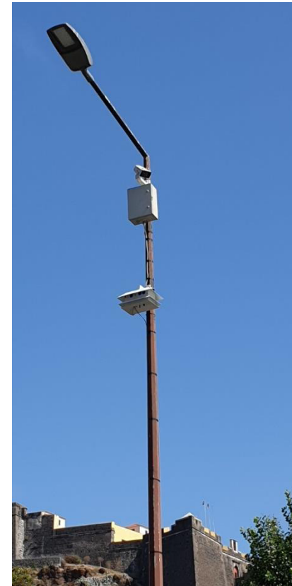
Environmental Monitoring Station in Madeira
