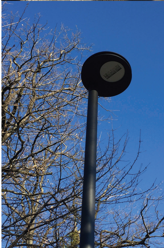
Figure 5: new luminaires with sensors&controllers (Park Vila Zora)
