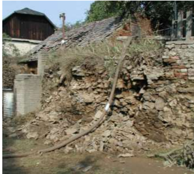
Destroyed retaining stone masonry wall constructed with clay mortar,.
