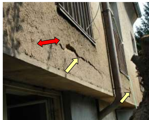
Parapet wall displaced by expanded floor beams.
