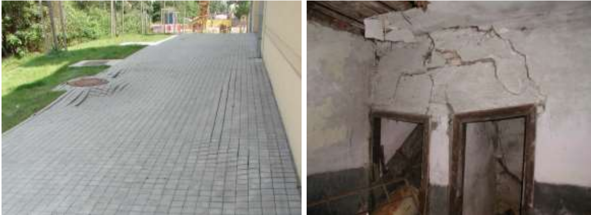
Left: Pavement deformation after flooding of infill made of collapsible soil; right: Partition wall deformation after additional compacting of washed away subsoil.
