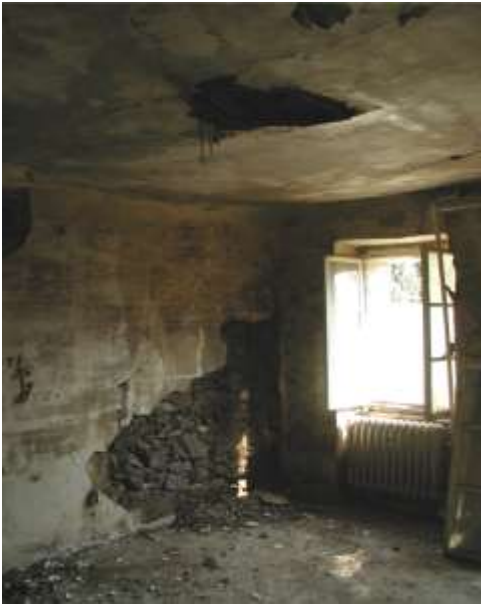
Washed out clay mortar from stone masonry wall with fragile plaster not able to protect the wall.
