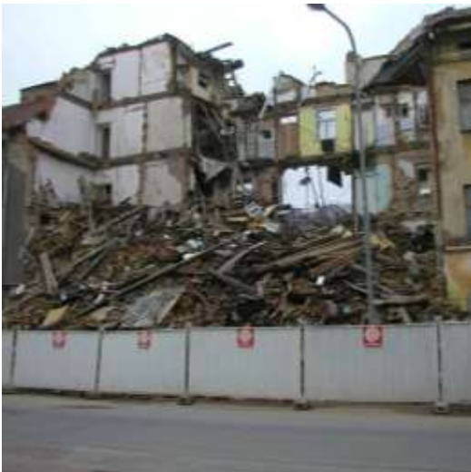
Failure of a dwelling house due to a loss of bearing capacity of brick masonry pillars.
