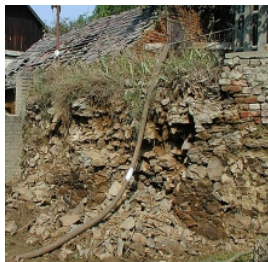
A destroyed stone-masonry retaining wall constructed with clay mortar.
