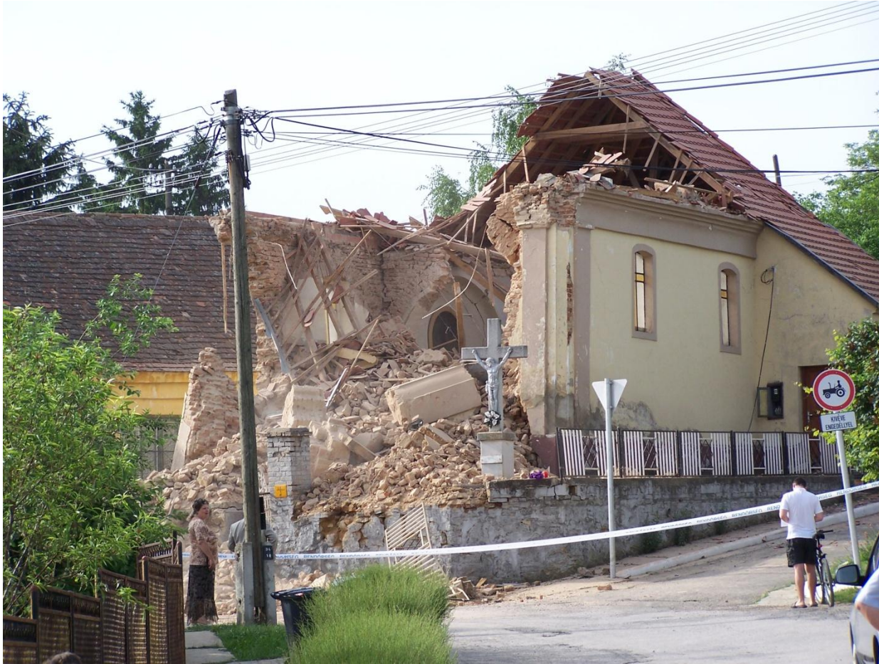
Collapse of the Roman Catholic church of Belvárdgyula, 2006
