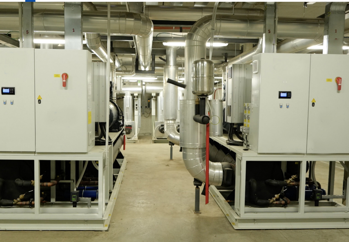
Chivasso Hospital - New refrigeration units
