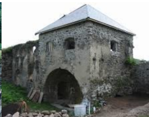
Figure 7 Gate no. II of Castle Čabrad' - restoration done by local civic association Rondel.
