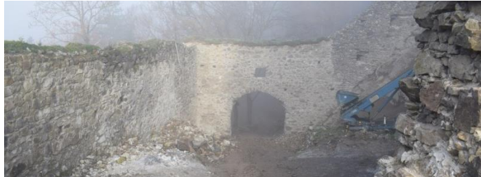
Figure 16 Restoration of the gate no. 1 and clean-up of rubble coming from a massive wall collapse into outer courtyard at Castle Revište
