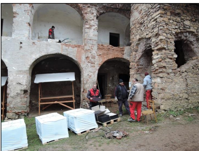
Figure 11 Non-qualified hands transporting material for roofing at manor of house Coburg in Jelšava.
