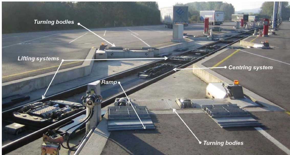
Figure 22. Specialized loading mechanism built into the transshipment track of Modalohr terminal Source: lohr.fr
