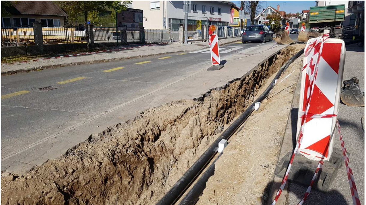
Figure 3: Pipes for district heating in front of the municipality building
