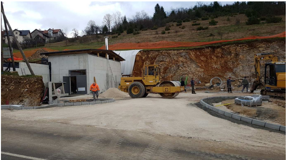
Figure 6: Boiler room, the first phase of a multipurpose facility that will be built until the end of 2018. Under the boiler room there is a 150 m 3 storage for wood chips.
