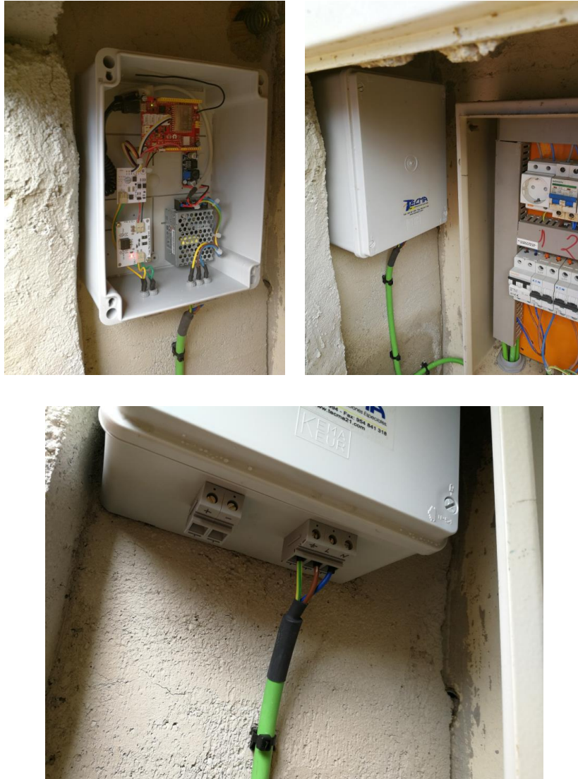
Figure 7. Lighting control module inside an outdoor switchboard, including the terminal prepared for the future connection of the DALI control bus.
