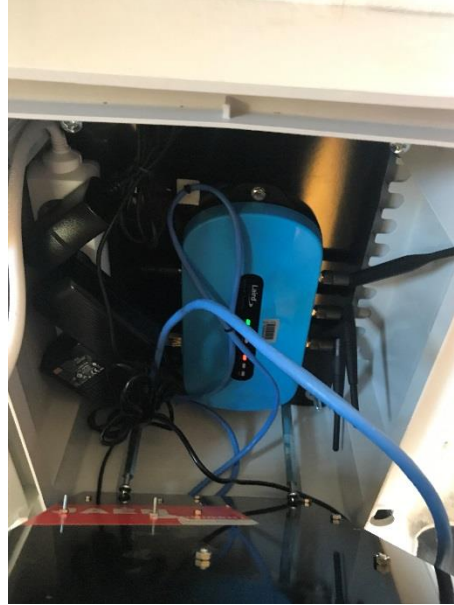
Figure 3. Gateway for communications between the lighting system and the management software.
