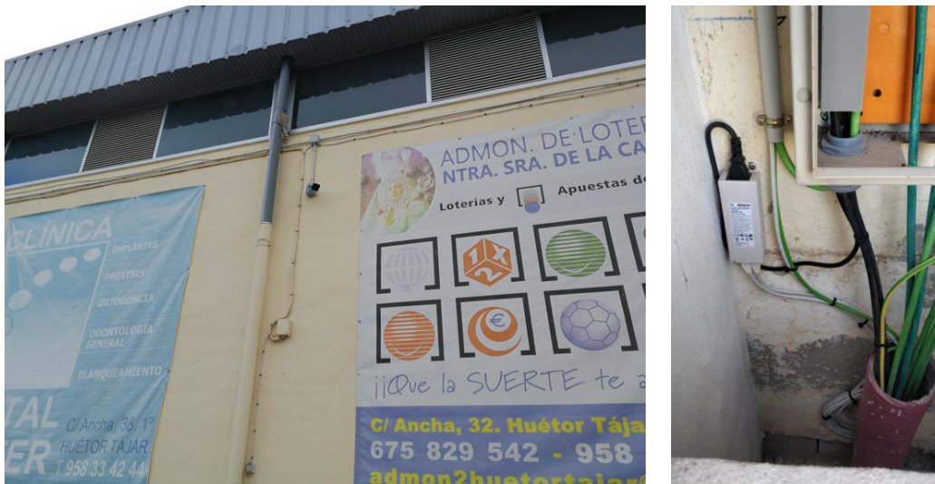
Figure 11. IP camera for people counting and its PoE injector inside one of the outdoor switchboards of the floodlights poles.
