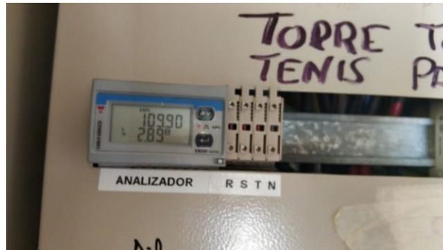
Figure 8. Power grid analysers and current transformer for the measurement of electrical variables.
