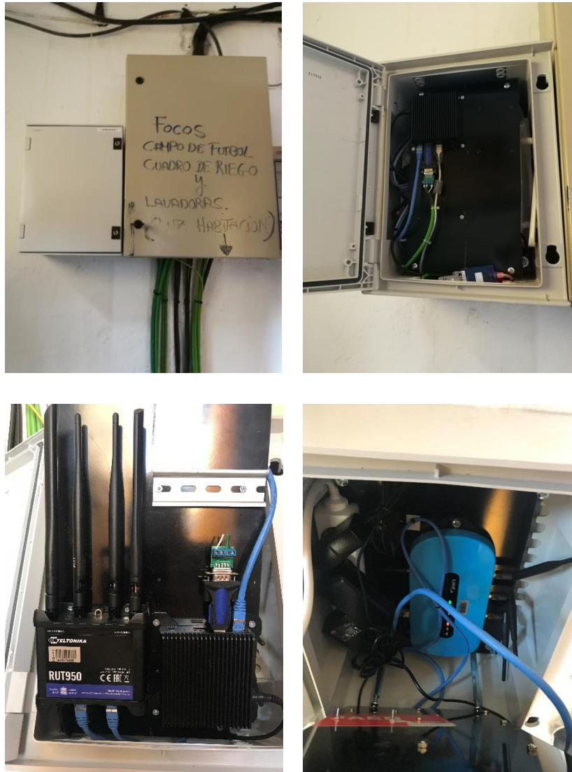
Figure 9. Switchboard installed to host the gateway, the mini PC and the 3G router, next to the main switchboard of the football pitch.
