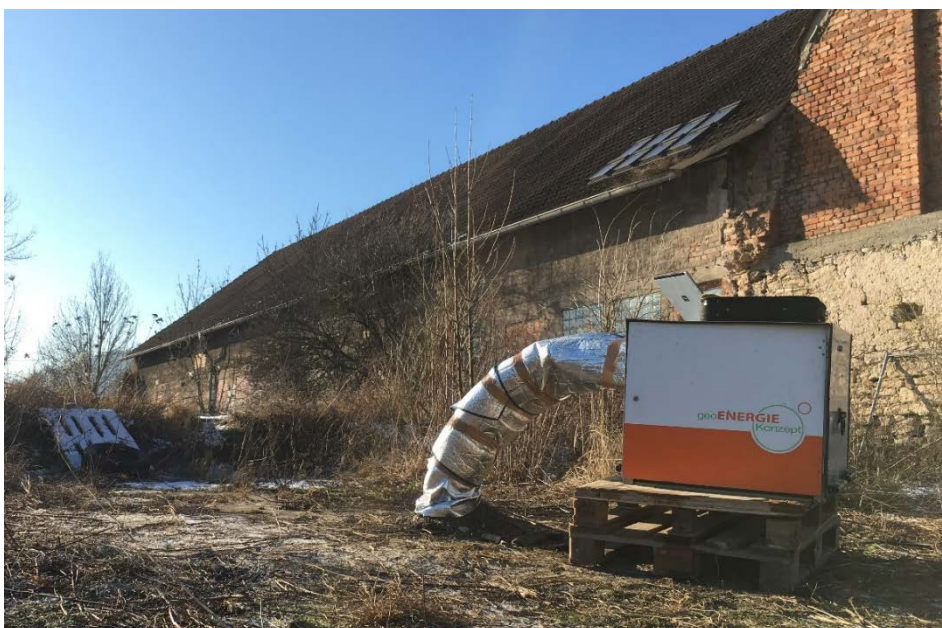
Figure 6: TRT Device #2 (PP03 - geoENERGIE Konzept GmbH).
