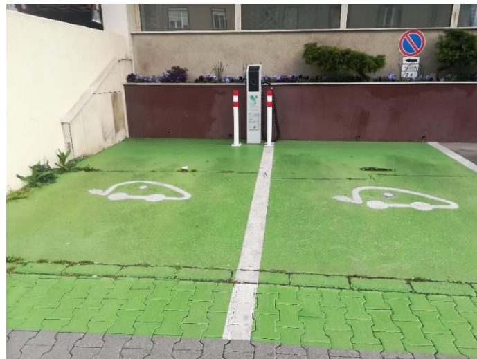
FIGURE 12: ELECTRIC CHARGING STATION NEXT TO THE CITY HALL OF DISTRICT 18
