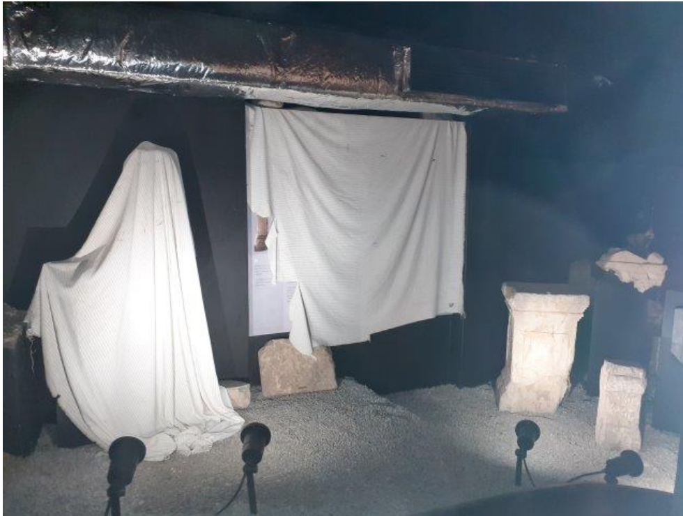
Figure 39 : Ventilation system inside the historical building 1
