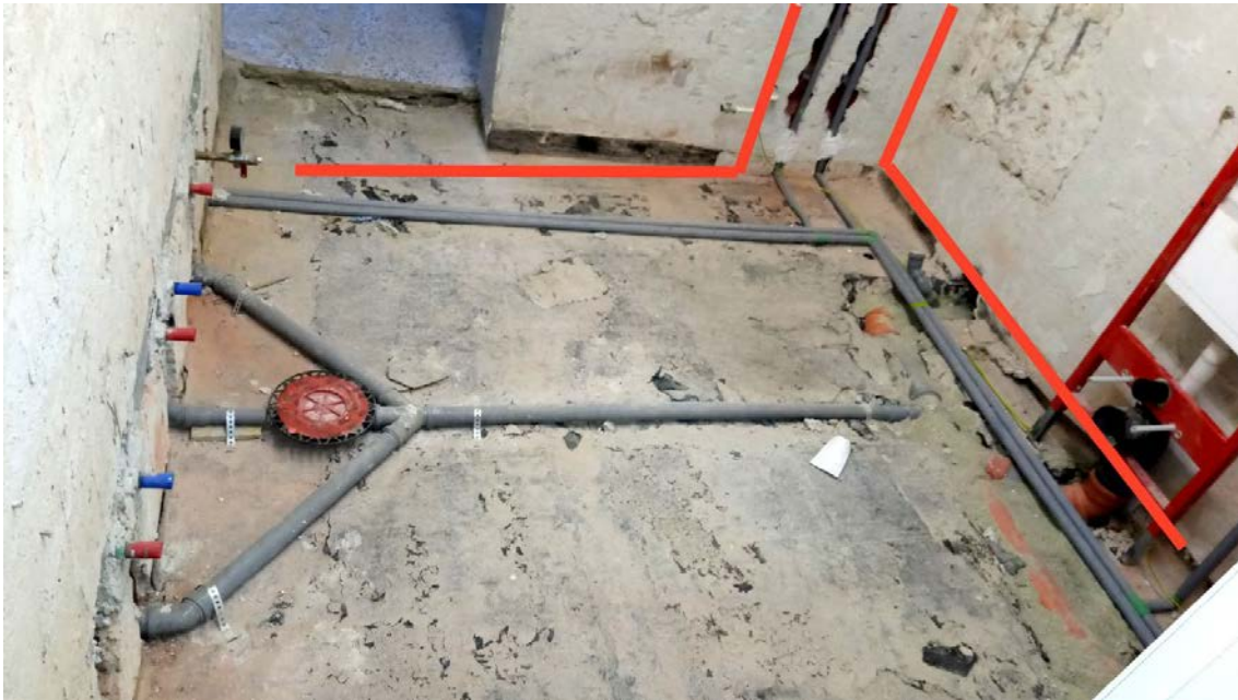
Figure 3 : ...the floor pipes in bathrooms.
