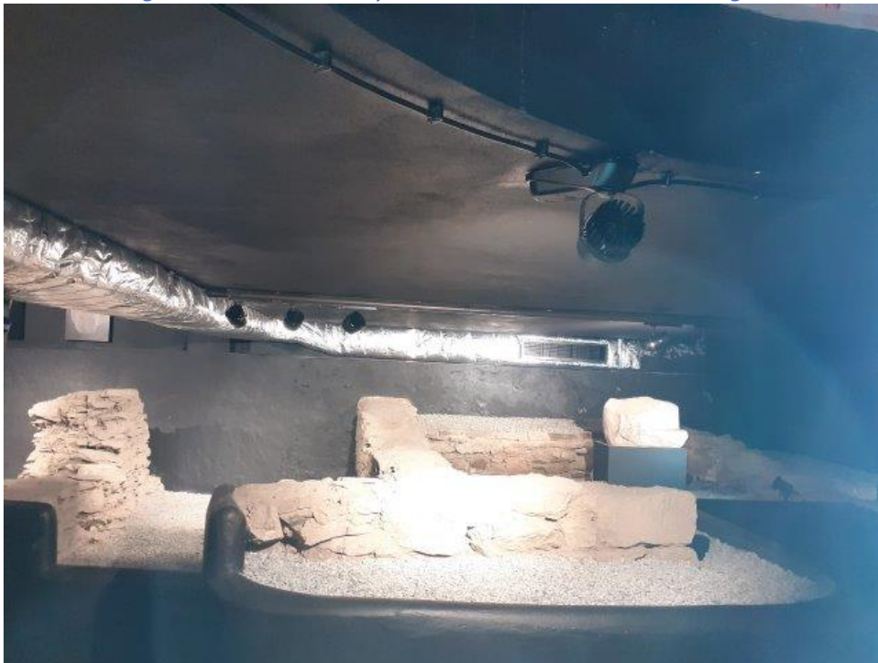
Figure 40 : Ventilation system inside the historical building 2
