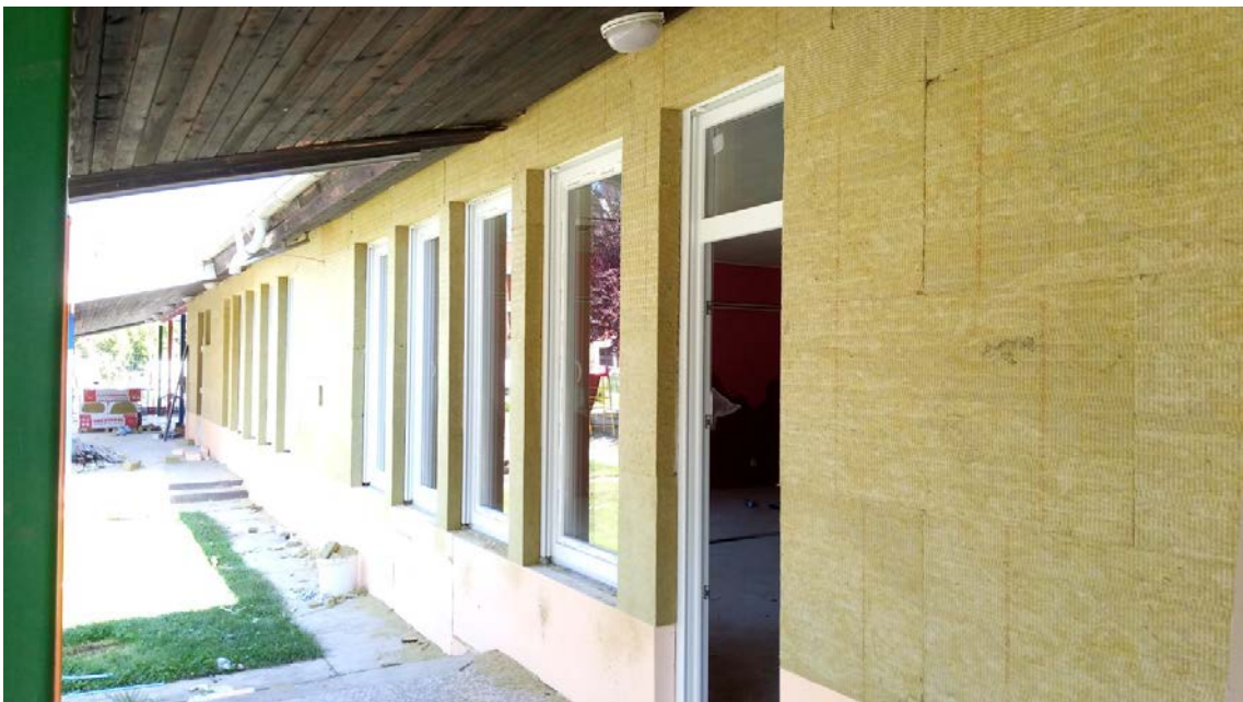
Figure 12 : Thicker-than-possible thermal insulation of walls
