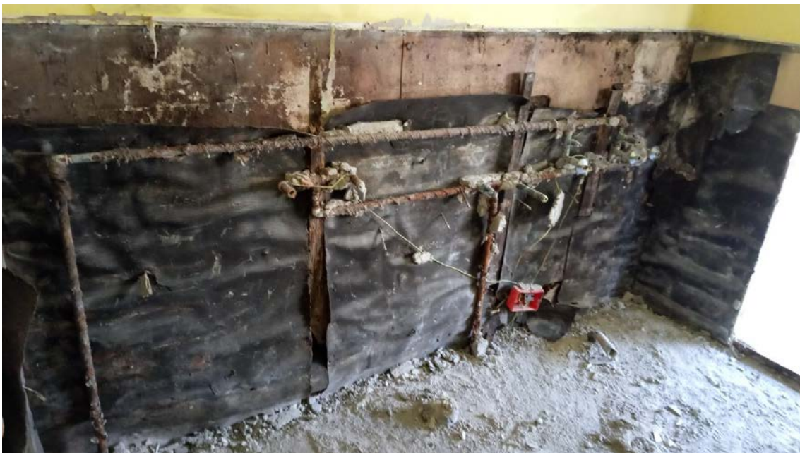
Figure 4 : Original outdated installations and walls in children bathrooms
