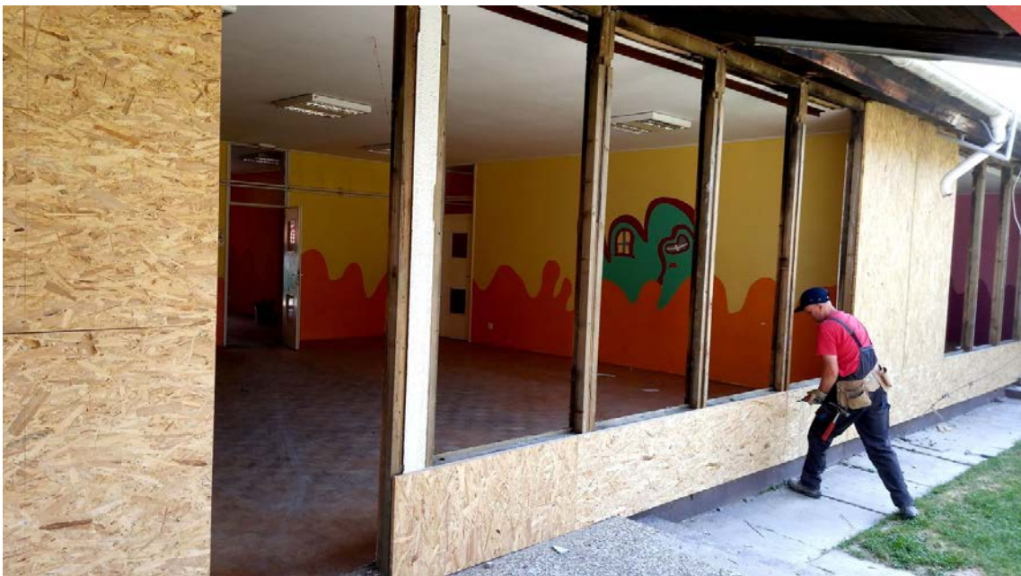
Figure 8 : Reinforcing the envelope with ordinary OSB panels in a complete new way
