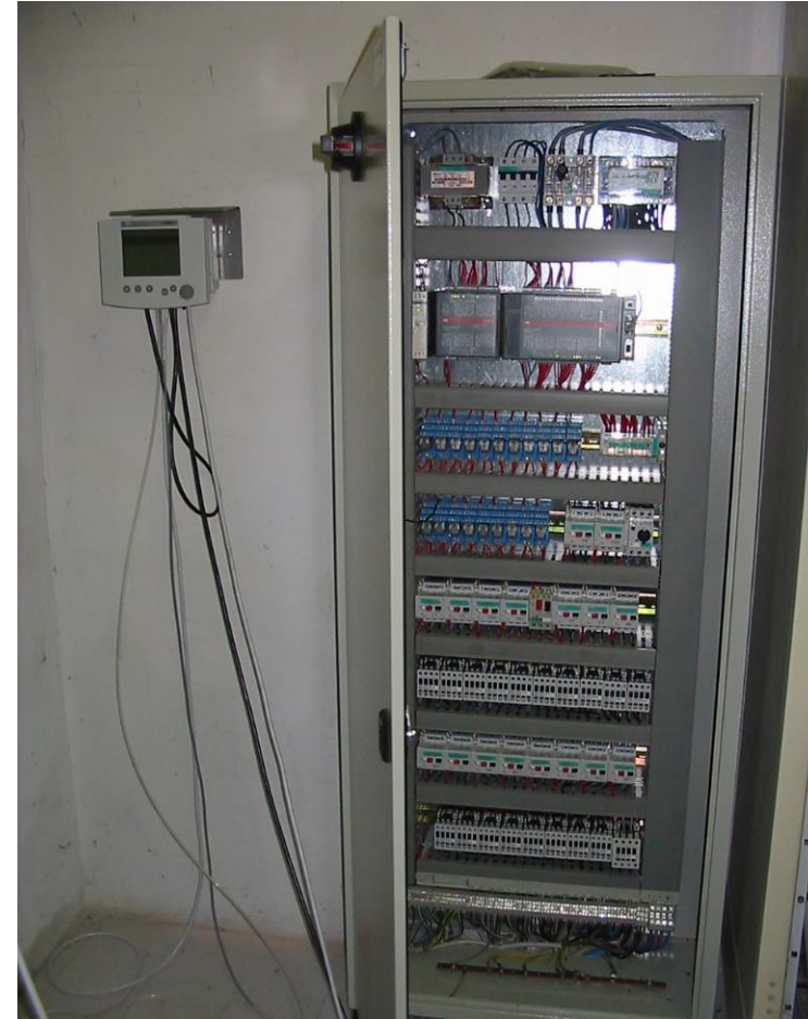
Electrical control panel
