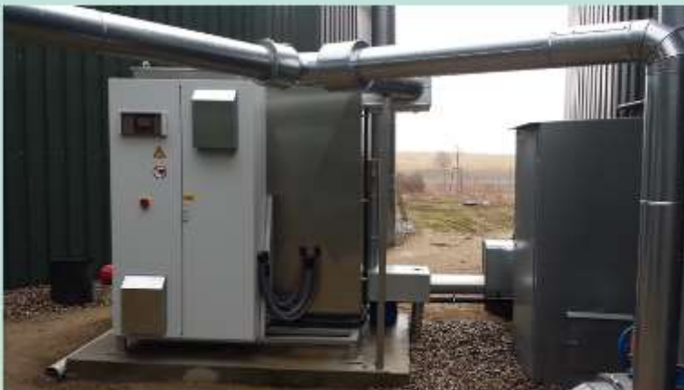
Göritz biogas plant: Wave-Box, treating second-step-digester medium, recirculation back to digester
