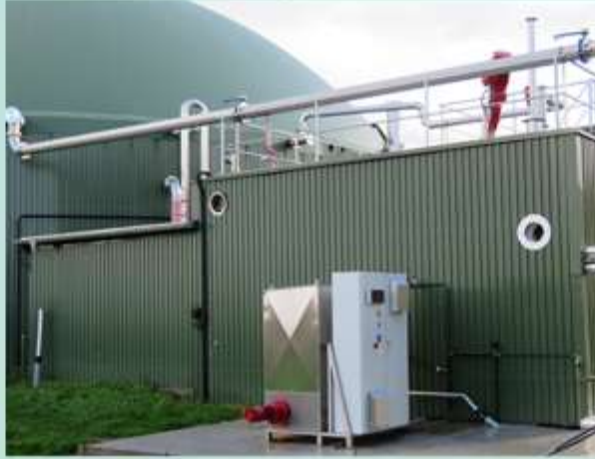
Wave-Box, treating second-step-digester medium, recirculating into Kombi-Hydrolysis
