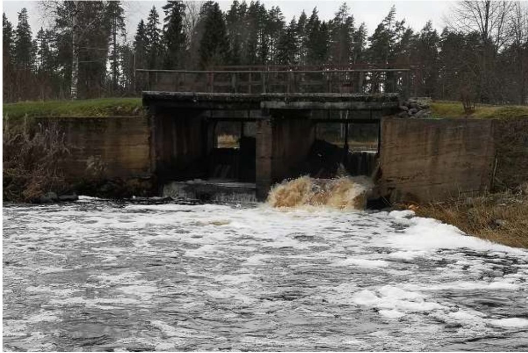
Photo 18. Dzirnavas dam's water level is raised by ca 2,1 meters. During high water some of the stoplogs are removed and therefore the expansion level is lower. On the day of the observation only the left excess water outlet was partly open which is achieved by removal of the stoplogs. Dam's owner is concerned with the unexpected openings of the Holdre dam, after which there is a risk of flooding in the Dzirnavas dam (R. Järvekülg, 08.12.2019).
