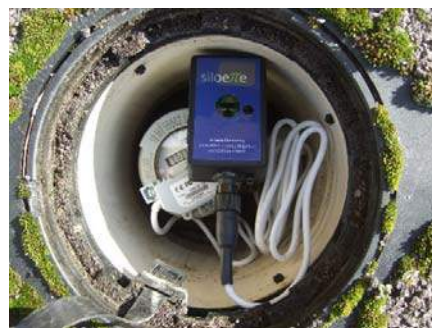
Fig.1. Siloette logger attached to water meter
