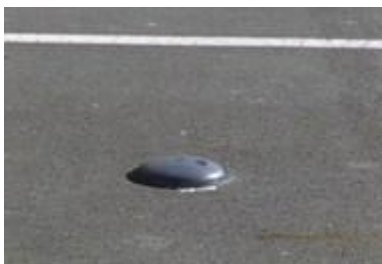
Figure 14: Example of an infrared detector installation, source: (12)
