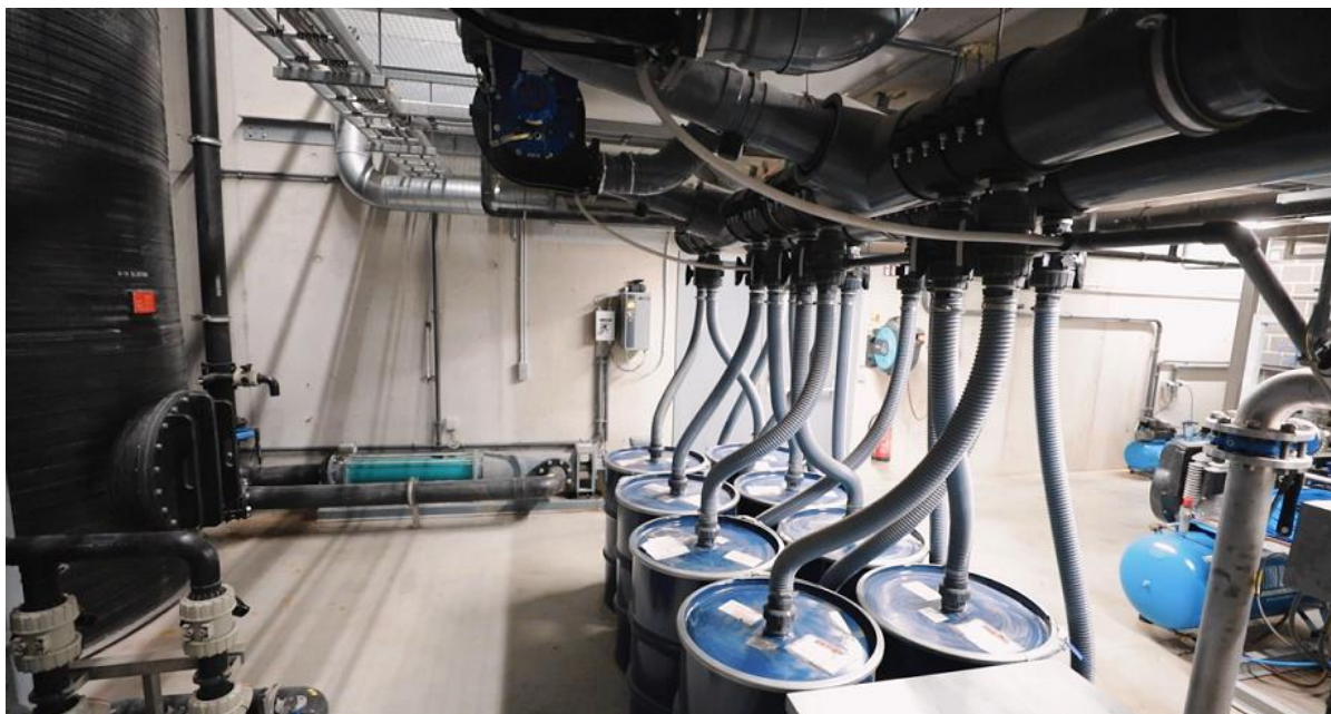
Figure 5 - DuCoop's wastewater treatment plant at De Nieuwe Dokken
