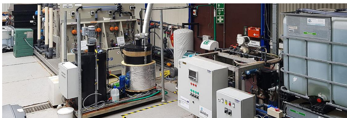
Figure 1 - Evides' pilot plant in Den Hoorn
