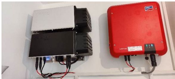
A battery storage system installed in a Rotterdam demo home.
