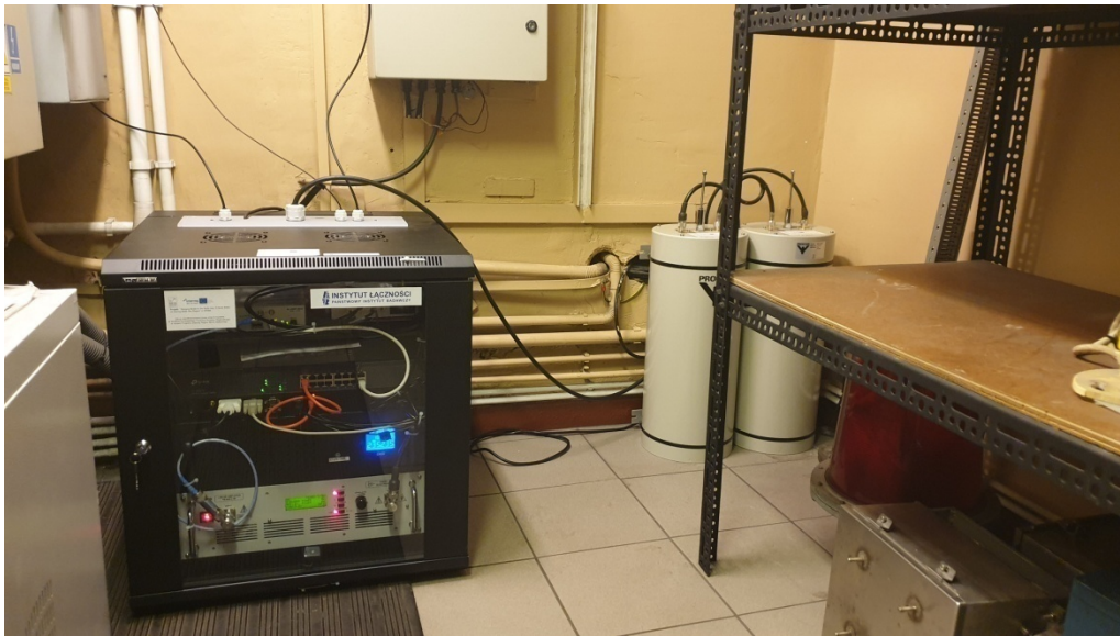
Figure 2-4: Designed R-Mode base station installed in the MOG spot in Port Gdynia
