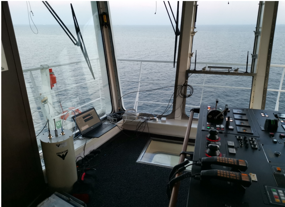
Figure 2-2: The receiving side of the measurement stand installed on the ferry
