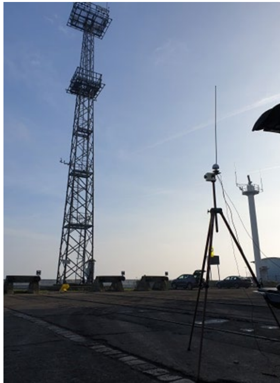
Figure 2-5: MOG tower with VHF antenna installation and a part of calibration stand
