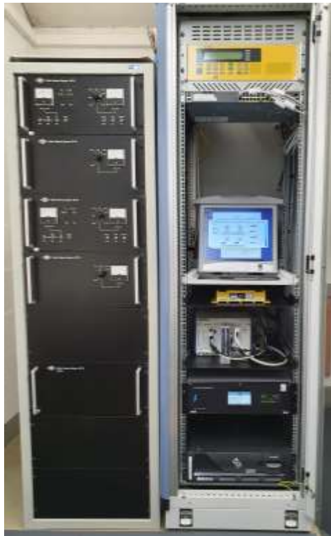
Figure 10 Typical R-Mode/DGNSS site in Germany
