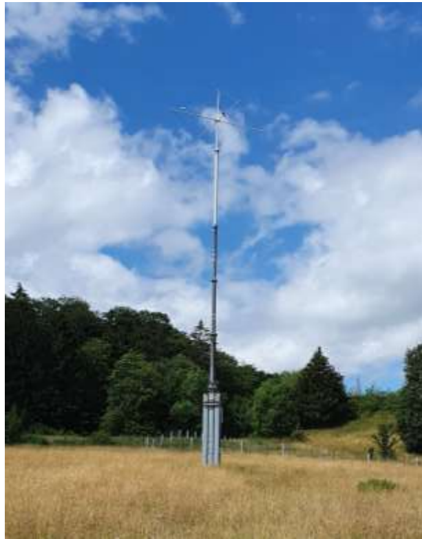
Figure 11 Typical MF antenna used on German R-Mode/DGNSS sites (Typ NTA, Koblenz DGNS)
