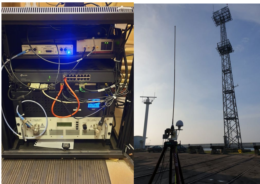
Fig. 6.3 Rack-mounted VDES R-Mode transmitter hardware and the 20m tower in the port of Gdynia
