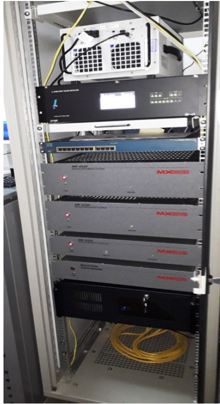
Fig. 3.3 Reference generator mounted in the rack at DGPS R-Mode Rozewie station, 2021.
