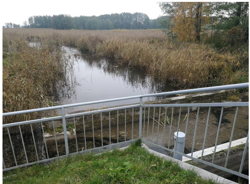
Figure 3. One of the spill-weirs in Metelytė (between Dusia lake and Simnas Fishery Ponds). Due to hydrological drought the water level is becoming dangerously low and at risk of not flowing through the weirs.
