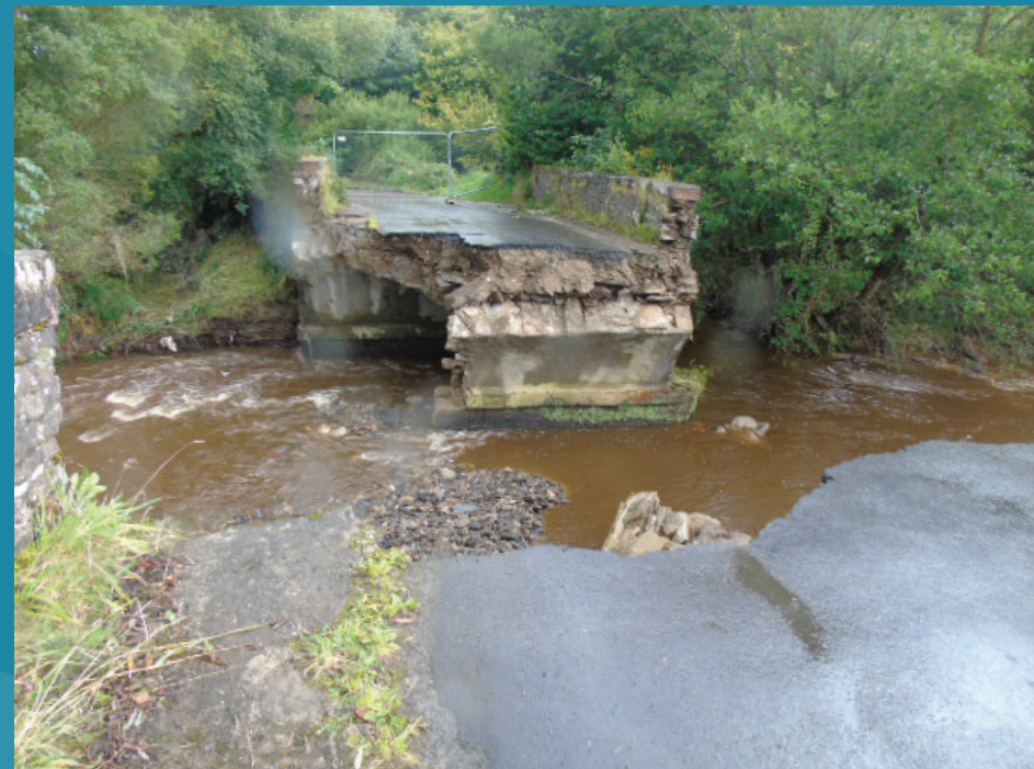
Bridge Collapse August 2017 Flood Event
