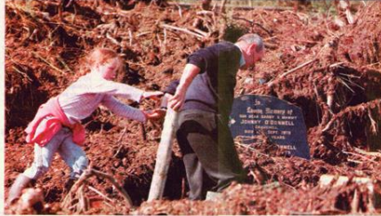
Pollathomas Graveyard which was destroyed by a landslide after torrential rain. Photo: Keith Heneghan / PHOCUS
